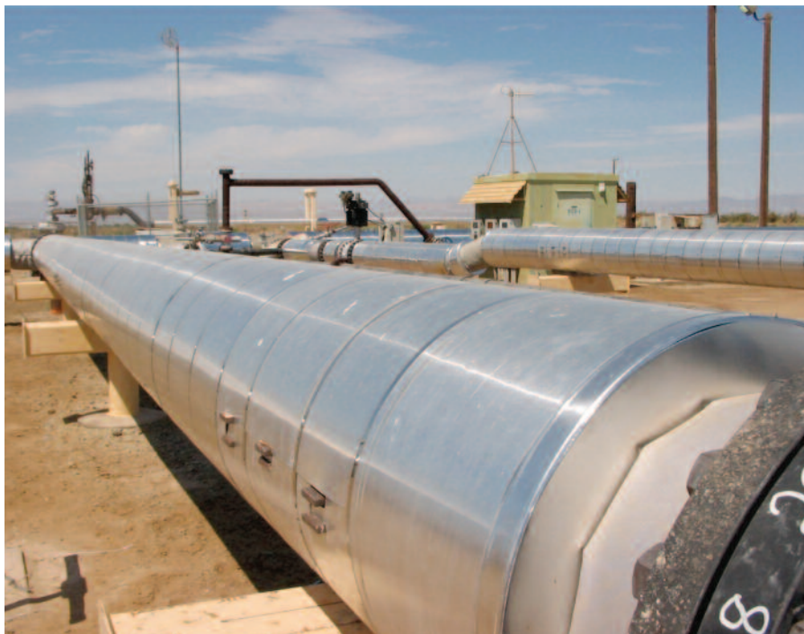
Super duplex 2507 turbine feed pipeline.
